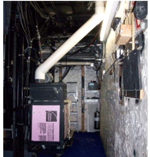
The basement trap room of NYC's Majestic Theatre is packed with automation and effects equipment
