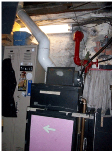
Another machine plumbed around the crew lockers
