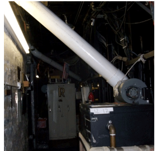
More of the six machines with 6" PVC pipe plumbing for sending fog to the stage
